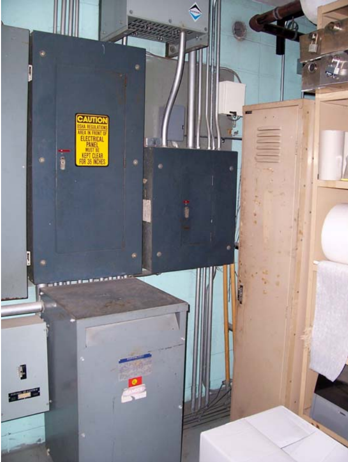
Photo 1-7 - 36" clearance required at electric panels.
